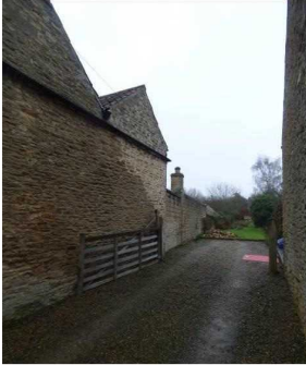
Further general view of west elevation to applicant's property. Note also applicants guttering which overhangs neighbour's property.
